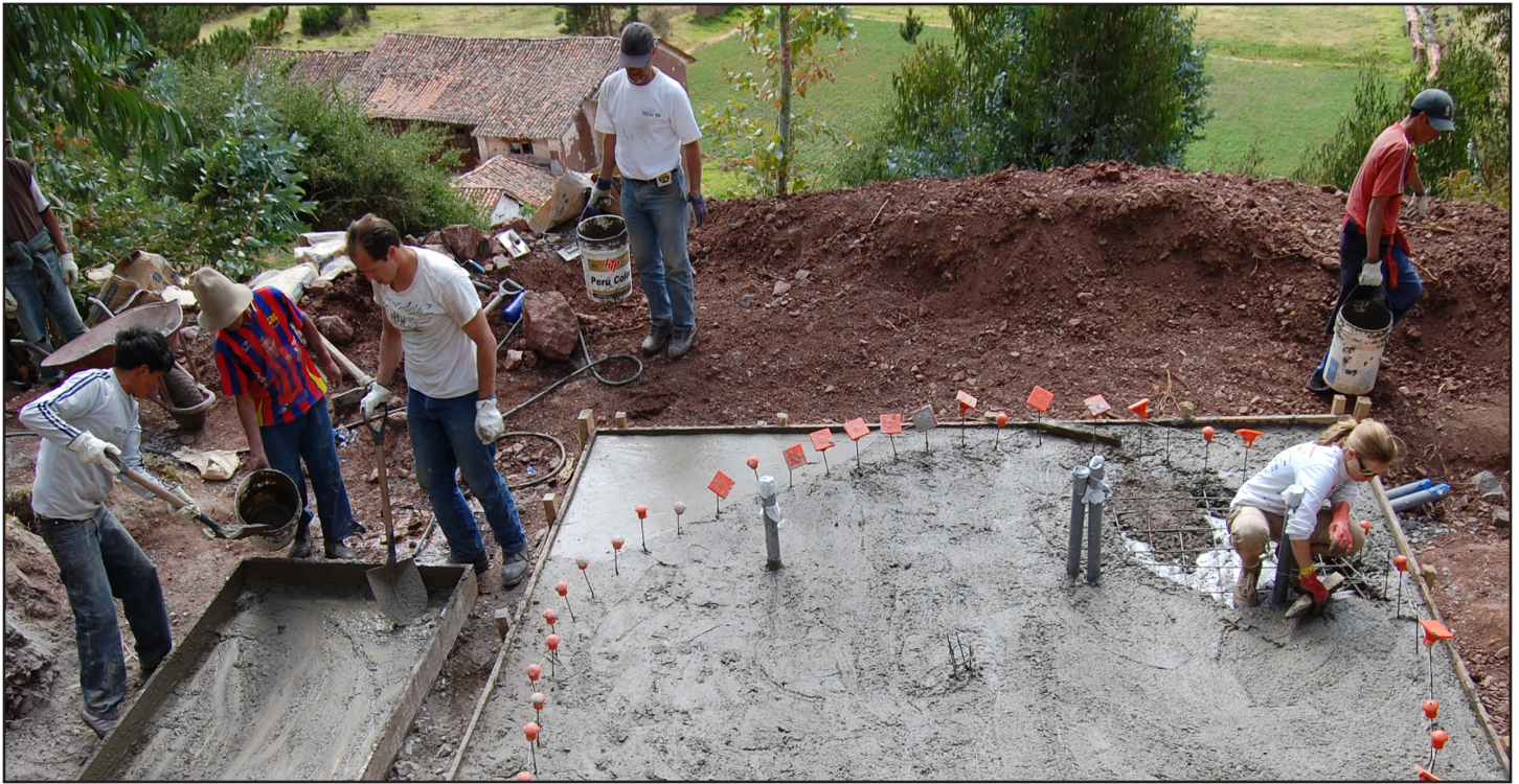
University of Maryland students Headley Jacobus and Keshi Jordan work with professional engineer John Sankey and community members of Ayotomibamba to mix concrete and lay the foundation for a new water tank.
