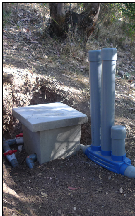
A chlorine dosing system that was installed by the EWB Peru Team
