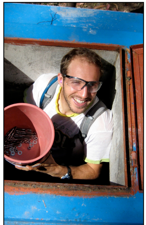
UMD Student Elliot Cohen enters a reservoir with the hardware necessary to install baffles.
